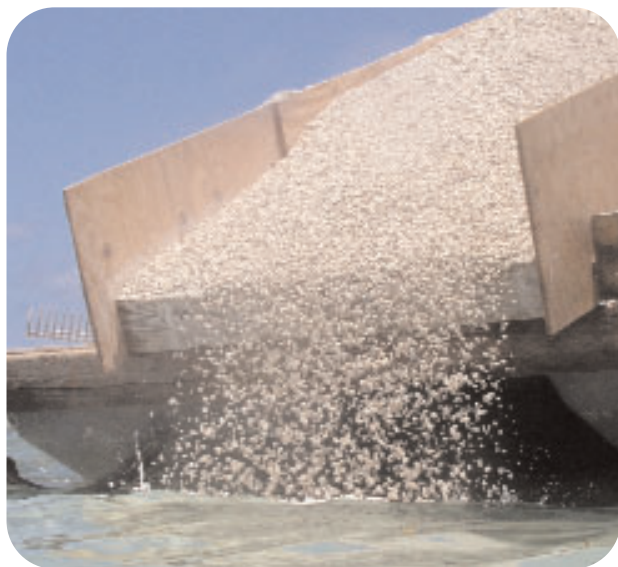
Pearock is poured from a barge to fill a blowhole. Deeper scars and blowholes must be filled because seagrass plants will not grow downward, away from the sun. (Photo: Alicia Farrer)
